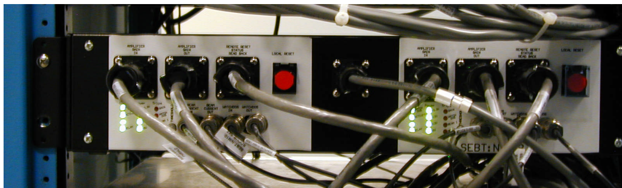
Figure 3. SEBT Non-Intercepting Monitors control box. Location: Row 1, Rack 7, ISAC-II Power Supply Room.
